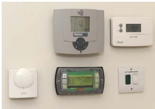
Figure 7: Heat pump and solar hot water controllers
