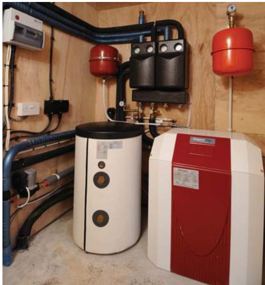
Figure 2: Ground source heat pump inside Energy Shed
